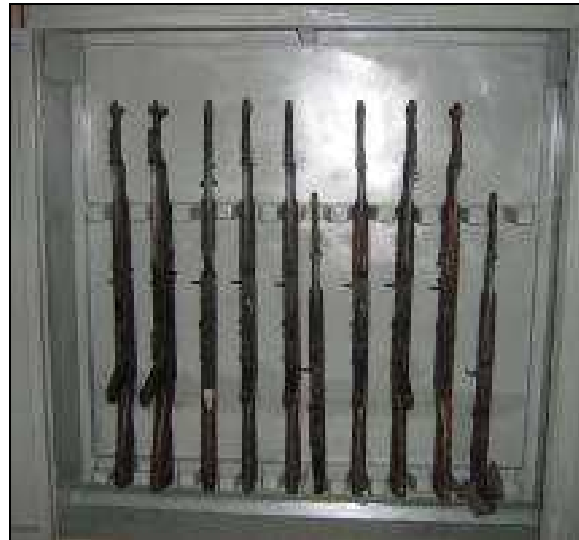
DRC: Prefabricated weapons cupboard as installed at Makala Prison in Kinshasa
