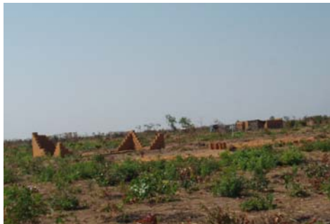
Houses being constructed on cleared land in 4 de Fevereiro This land was cleared during the previous quarter and the speed at which it is being occupied by families illustrates the demand for land for returnees.
